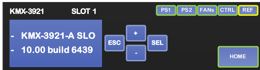
CPU-ETH3 local control panel
