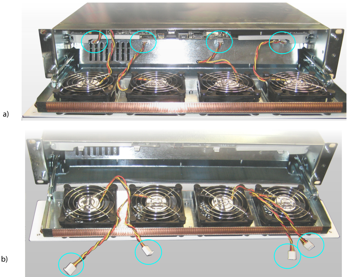
Fig. 6-8: Door-Fan Supply Wires: a) Fan Wires Connected to MV-821 Main Module. b) Fan Wires Disconnected.
