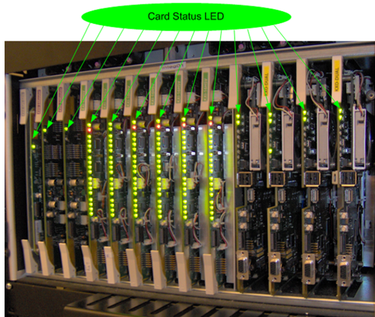
Photograph of a Kaleido-X (7RU) frame showing LED indicators on modules.
