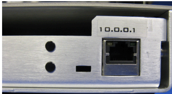
Figure 8. Monitoring Ethernet Port
