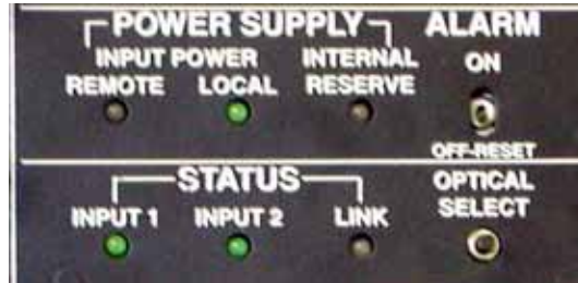
Figure 19: Panel Indicators, Signal Status and Power
